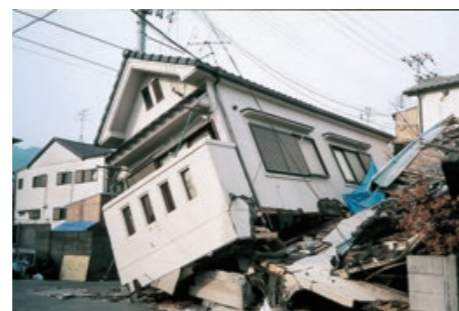
A house destroyed in the Great Hanshin-Awaji Earthquake, photographed by Professor Kenji Miyazawa
